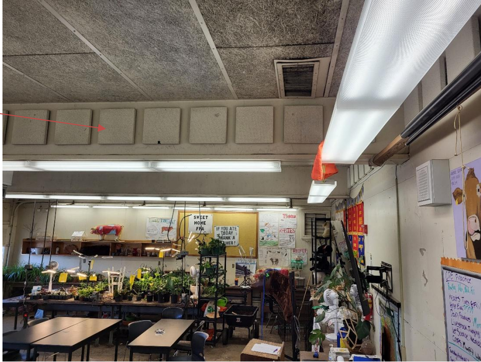
Photo 3 – D1: Brown Mastic Glue Dots (Behind Decorative Tiles) = 2% Chrysotile Asbestos
