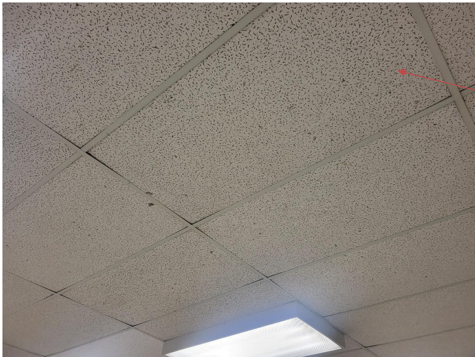
Photo 16 – A Building (East Block): 2'x4' Drop Ceiling Tiles = 2% Chrysotile Asbestos
