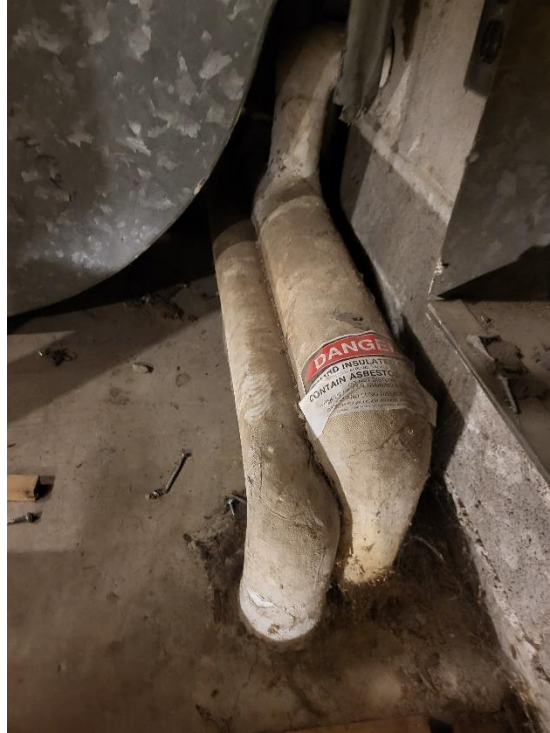
Photo 7 – Building B Mechanical Room: Hard Fittings = Asbestos Containing Material
