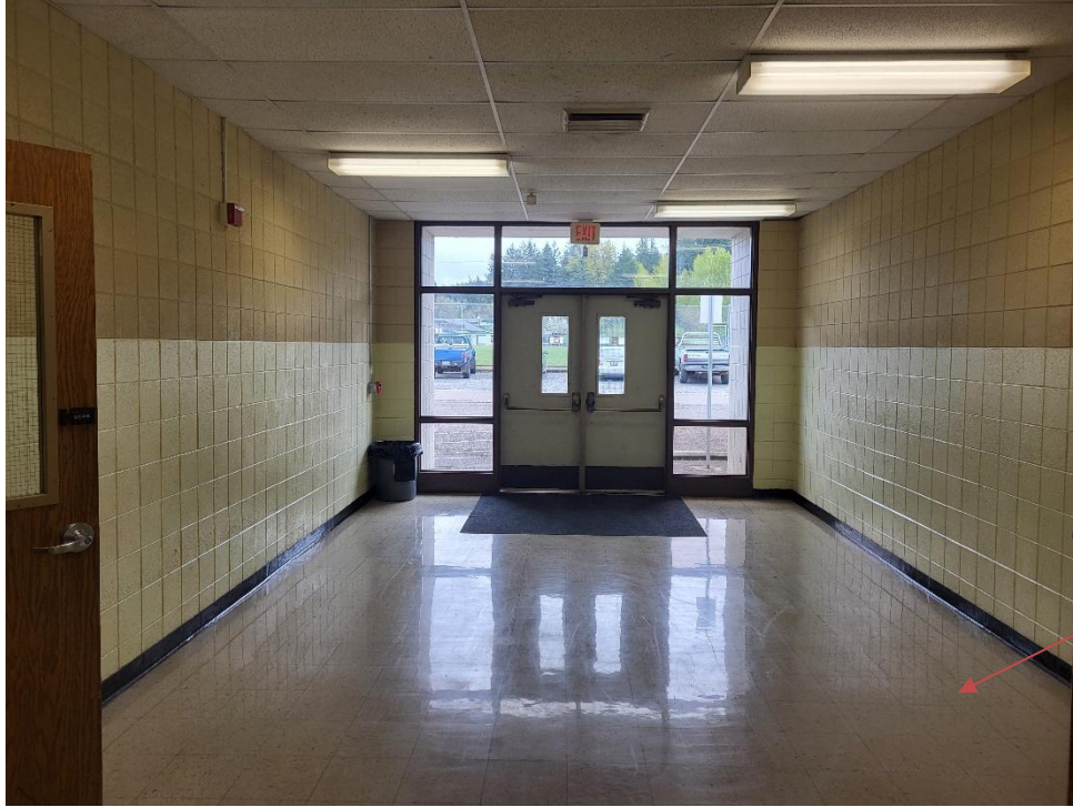
Photo 13 – C Building: Beige 12"x12" Vinyl Floor Tiles with Black Mastic = 3-4% Chrysotile Asbestos
