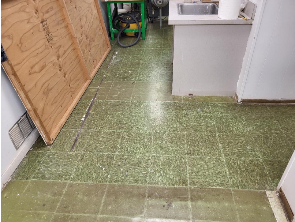
Photo 1 – D5: 12"x12" Green Vinyl Floor Tiles with Black Mastic = 3% Chrysotile Asbestos
