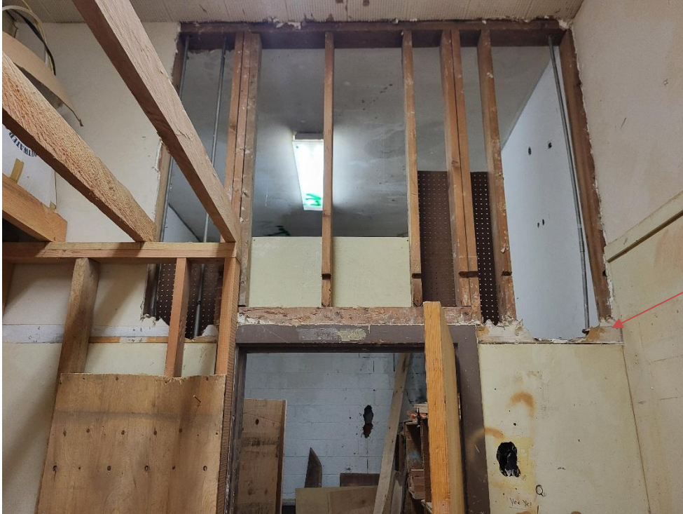
Photo 11 – Wood Shop Storage Room: Gypsum Wallboard with Joint Compound & Black Wall Mastic = 2% Chrysotile Asbestos
