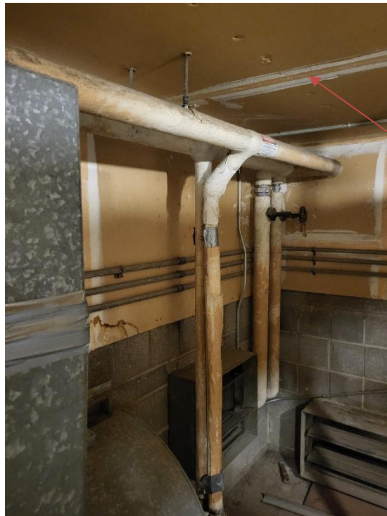
Photo 8 – Building B and C Mechanical Rooms: Gypsum Wallboard with Joint Compound = 2% Chrysotile Asbestos
