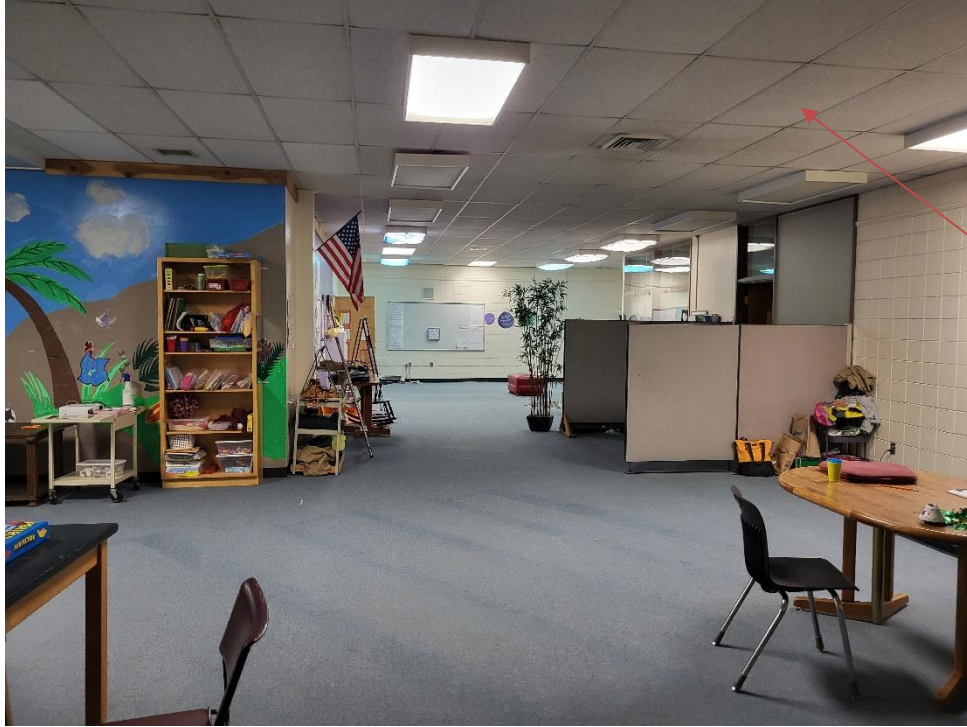
Photo 15 – B Building: 2'x4' Drop Ceiling Tiles = 2% Chrysotile Asbestos
