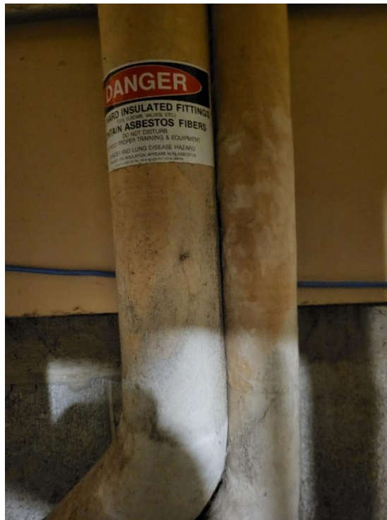
Photo 6 – Building B Mechanical Room: Hard Fittings = Asbestos Containing Material
