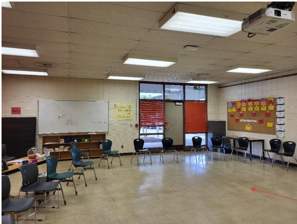
Photo 14 – B Building: Beige 12"x12" Vinyl Floor Tiles with Black Mastic = 2-4% Chrysotile Asbestos
