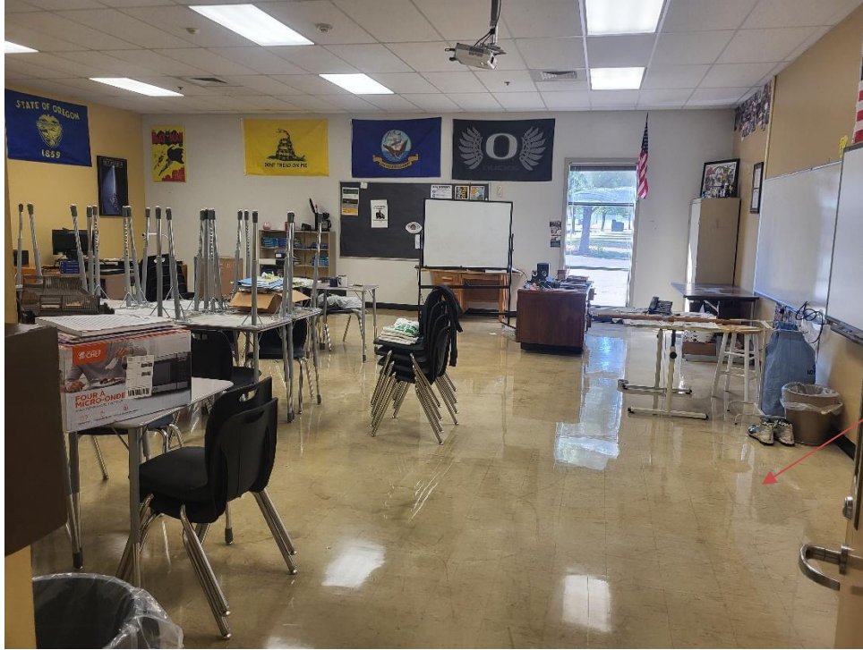
Photo 17 – A16: 9"x9" Vinyl Floor Tiles with Black Mastic = 8% Chrysotile Asbestos
