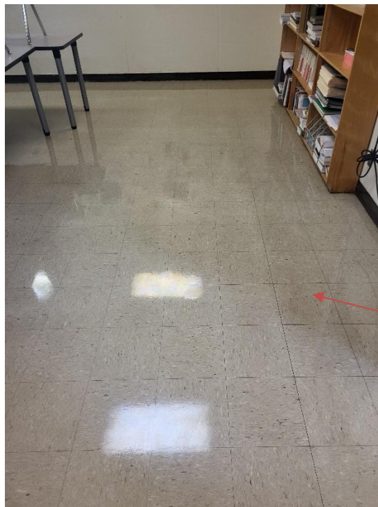
Photo 18 – A24: 9"x9" Vinyl Floor Tiles with Black Mastic = 3-5% Chrysotile Asbestos
