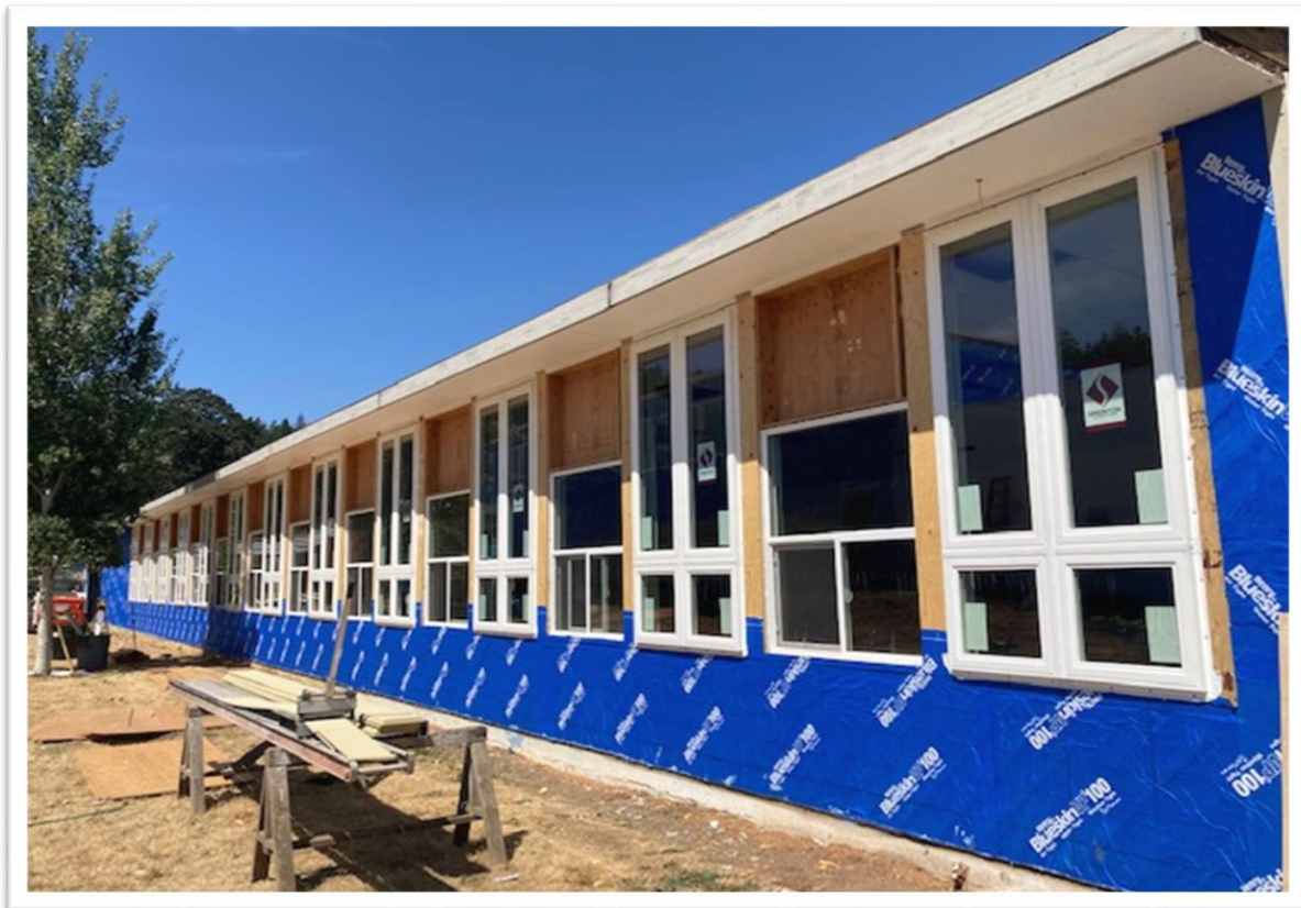
Construction work during the summer of 2024 on the Oak Heights Elementary School seismic project. Numerous improvements were made using District funds in addition to the grant funded seismic work.
