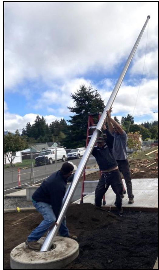
The Sweet Home School District facilities team installs a new flagpole at Oak Heights Elementary School, one of numerous improvements made at the school this past year.
