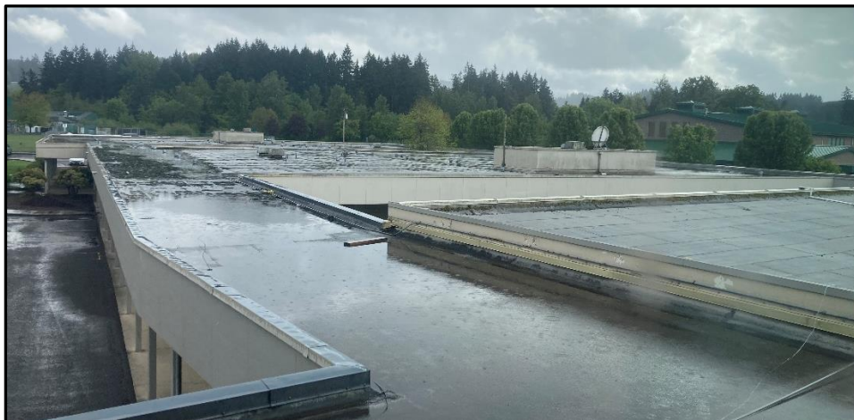
Puddles expand in size across flat-roof classrooms and nearby breezeways at Sweet Home High School as a spring shower passes through.
